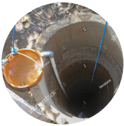
Borehole and Electric Pump
