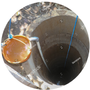
Borehole and Electric Pump
